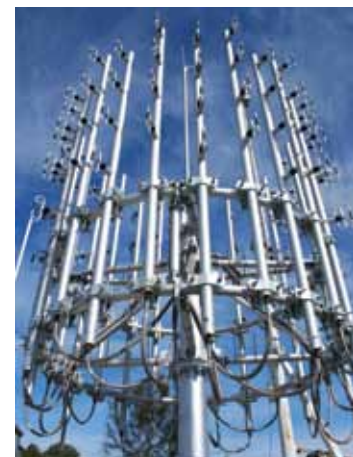
Ngara technology - Access Stage 2 Antenna Array.
